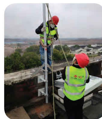
Network deployment at Huoshenshan Hospital
